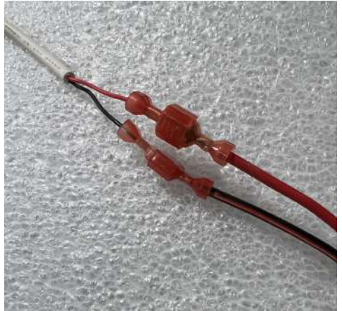
Low Voltage Lighting, Supply Connection
