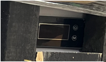
HEAT PUMP CONTROL PANEL
