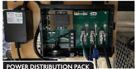
POWER DISTRIBUTION PACK
